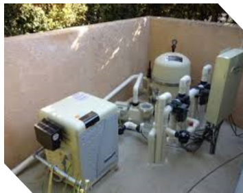
Figure 20: Pump and filtration system
