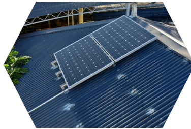
Solar PV array of 2 X 250 W for Direct DC electrical booster fitted on steel roof protecting concrete roof. Solar PV array of 2 X 250 W for Direct DC electrical booster fitted on steel roof protecting concrete roof.
